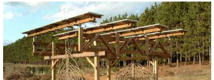
Wood PVOLT (PV Overhead Linkage Tracker) during 2001 demonstration installation
